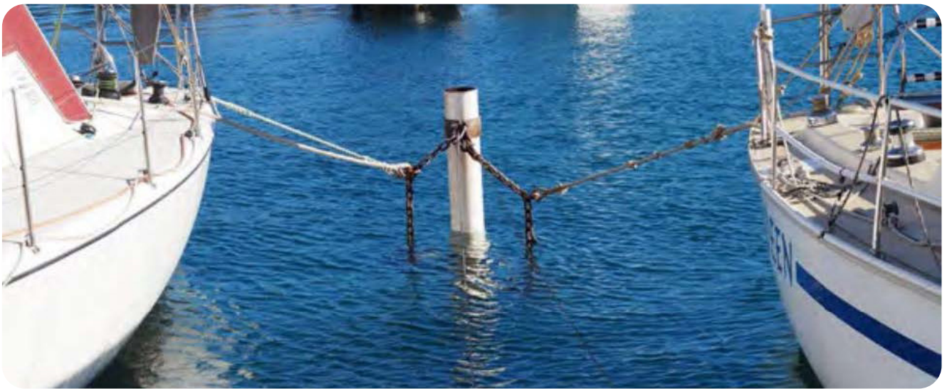
Marina Image 3 – undersized pylon with an open top end, this will allow corrosion to occur on the inside of the pylon which will not be able to be observed and monitored.
