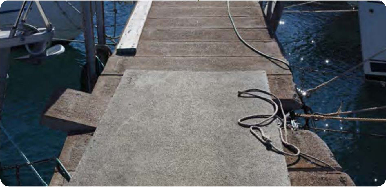
Marina Image 1 – Damaged walkway and improvised remedy. This timber piece, when wet, is not flat and poses a potential trip hazard. There is additional pressure on the substructure with uneven weight distribution.
