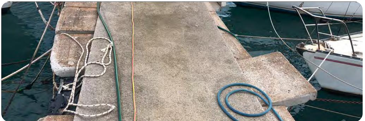
The existing Marina has a concrete deck, in this instance the slab has moved sufficiently to become a major safety concern and require remedial action. (October 2018)
