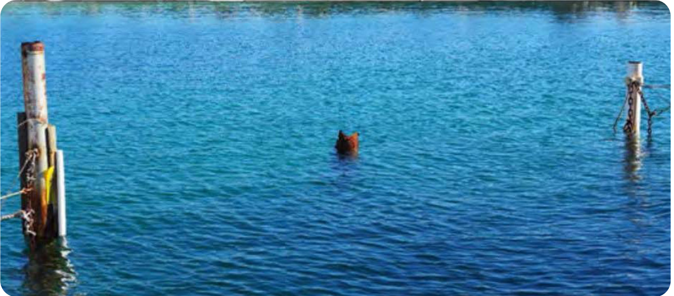
Marina Image 2 – Damaged pylon from corrosion, the two yachts had to relocate due to probable damage with approaching weather fronts. The two smaller pylons on each side are undersized and the top is open to the weather. The bracket on the right-hand side pylon poses a significant danger to the vessels departing and entering these berths.
