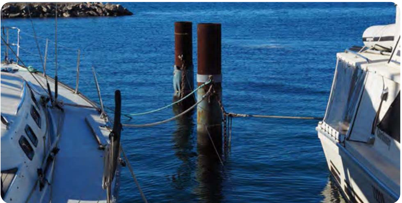
Marina Image 4 – larger pylons used to accommodate the larger vessels. Note these pylons are open ended and do not have any protection from corrosion.
