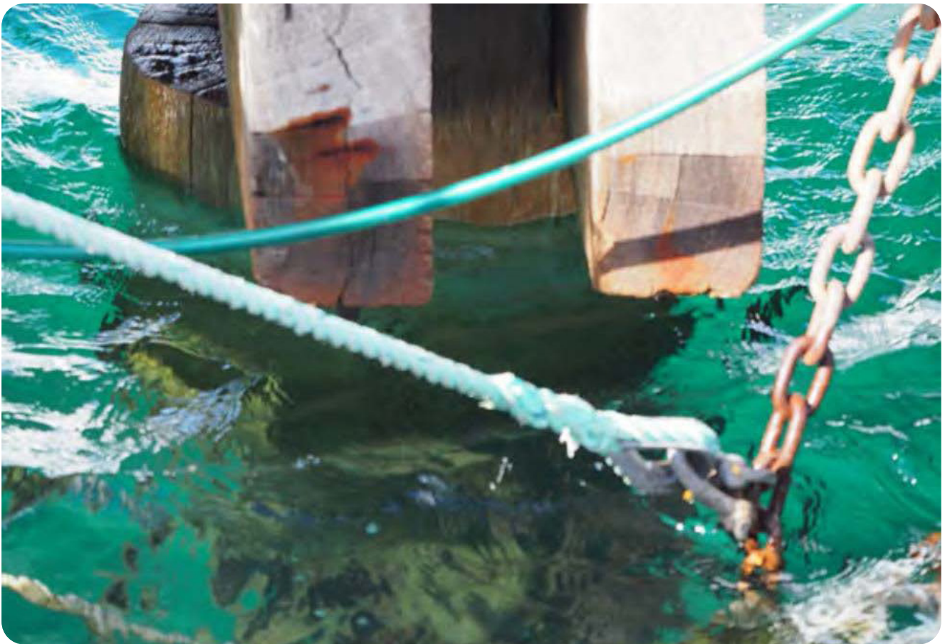
Marina Image 5 – timber pylon still in use, these pylons are subject to worm infestation and have probably been in situ for some 30 years. Their load carrying capability should be questioned.
